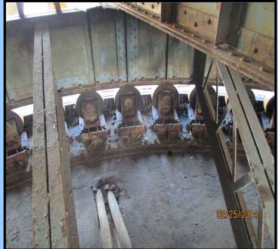
Photo 26: Swing span drum girders and machinery radial support beams, moderate rusting
