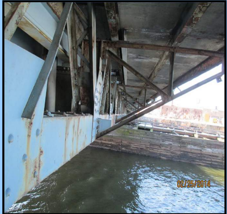
Photo 18: Severe rusting and localized section loss of steel stringers supporting sidewalk in swing span
