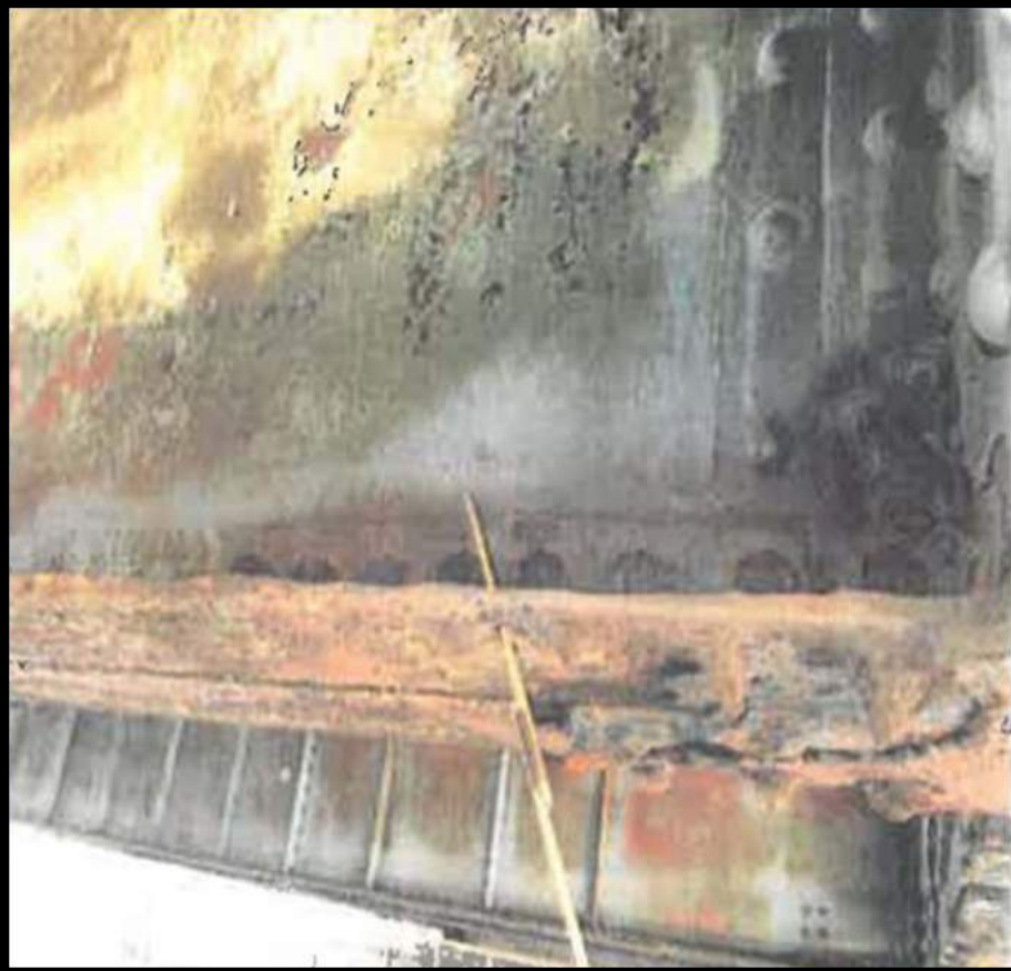
Photo 15: Severe rusting and hole in bottom flange angle leg of floor beam (FB12) of swing span
