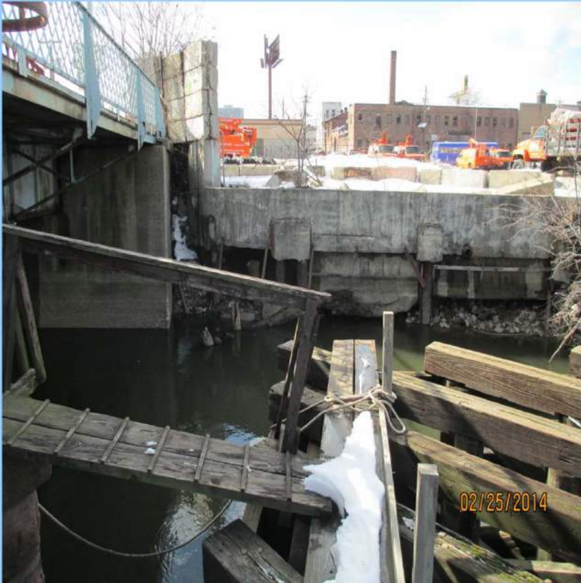
Photo 23: Northwest approach embankment undermining
