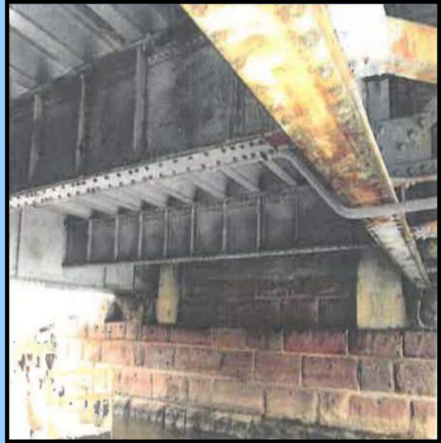
Photo 20: Rusting and localized section loss in girders and floor beams of west approach span
