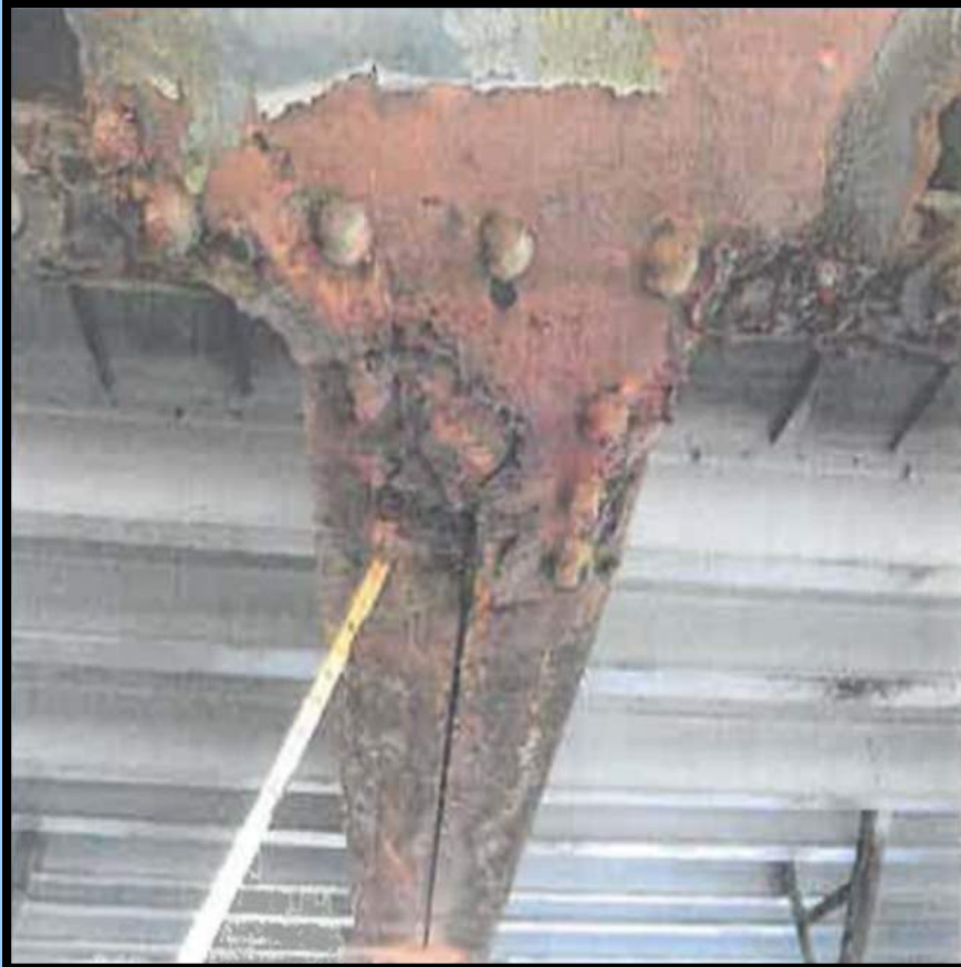
Photo 7: South truss bottom chord , severe deterioration to gusset plate, heavy rust throughout connection
