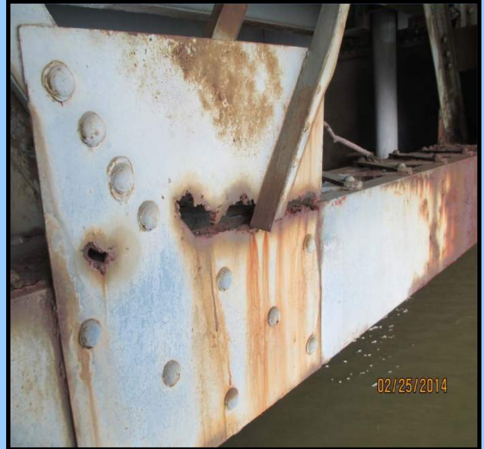
Photo 8: South truss gusset plate, severe rust with section loss
