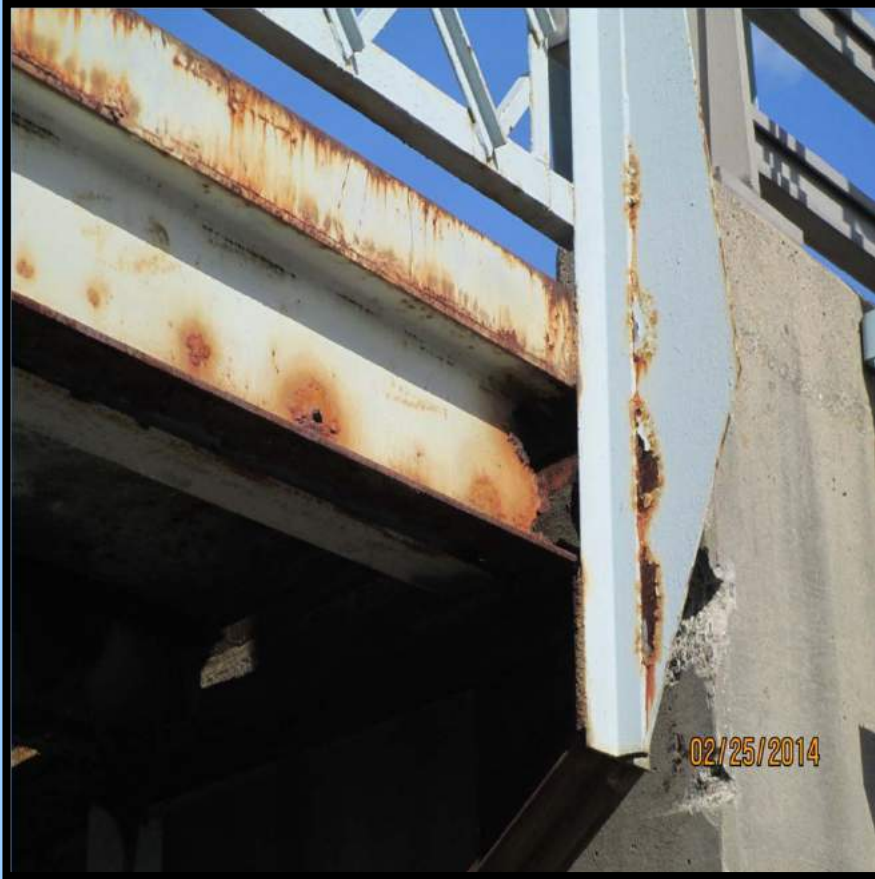
Photo 19: Hole in exterior girder of west approach span
