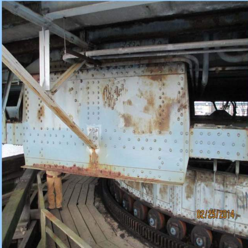
Photo 25: Rim bearing assembly of swing span – fair condition with corrosion build on exposed surfaces
