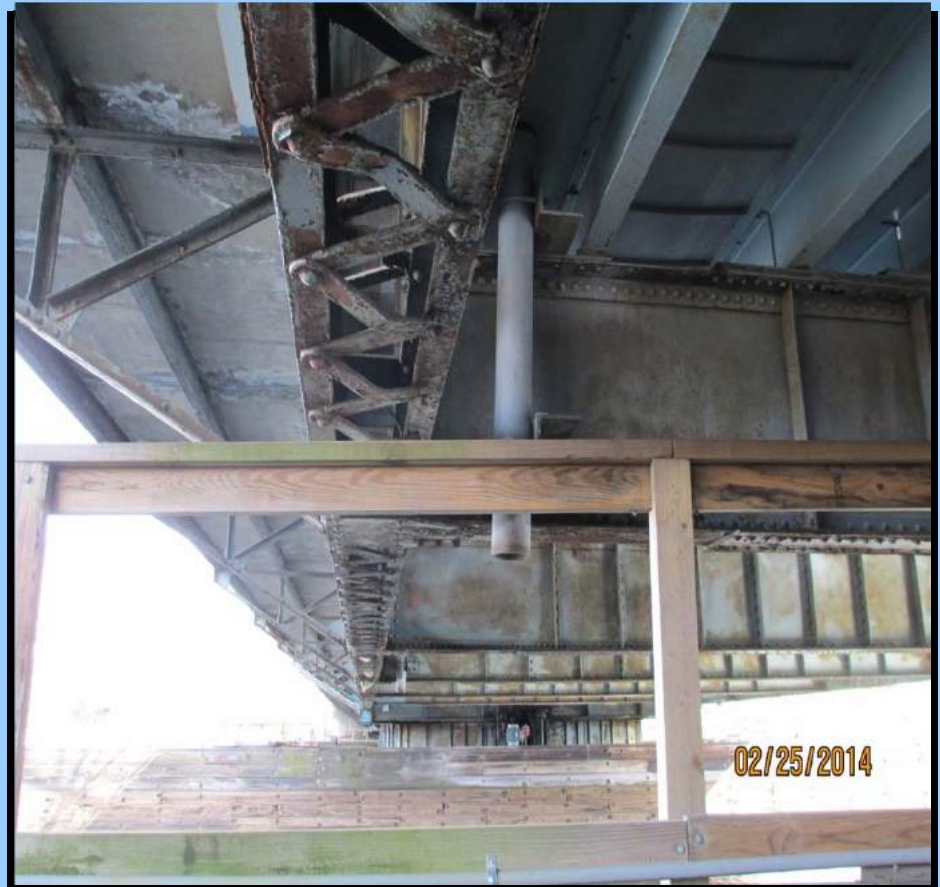
Photo 14: Bottom chord of south truss –severe rusting and localized section loss
