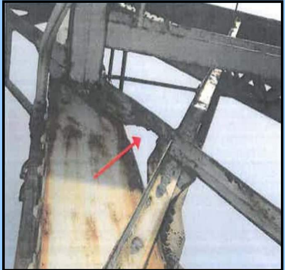
Photo 12: North truss; section loss in angle leg of member
