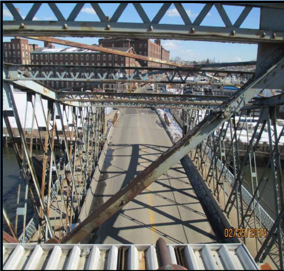
Photo 13: Localized rusting and material loss to top chords and diagonal truss members
