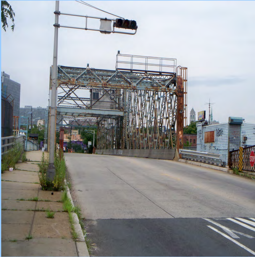
Photo 3: East approach to bridge looking west, substandard vertical curb
