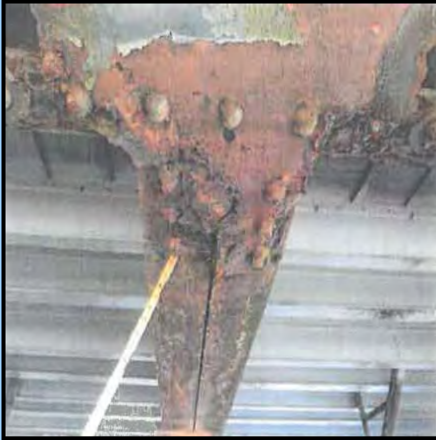
Photo 9: South truss bottom chord , severe deterioration to gusset plate, heavy rust throughout connection
