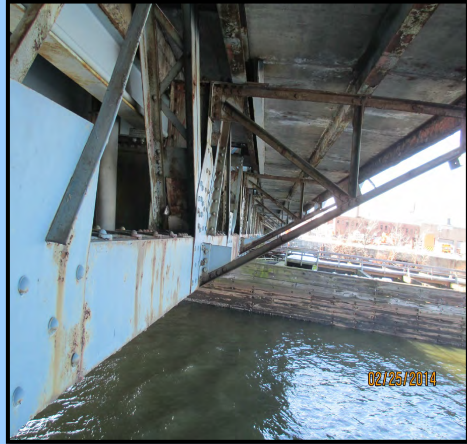
Photo 18: Severe rusting and localized section loss of steel stringers supporting sidewalk in swing span
