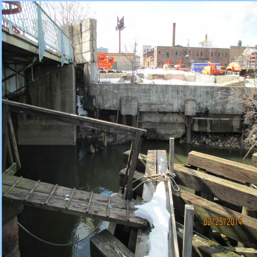
Photo 23: Northwest approach embankment undermining
