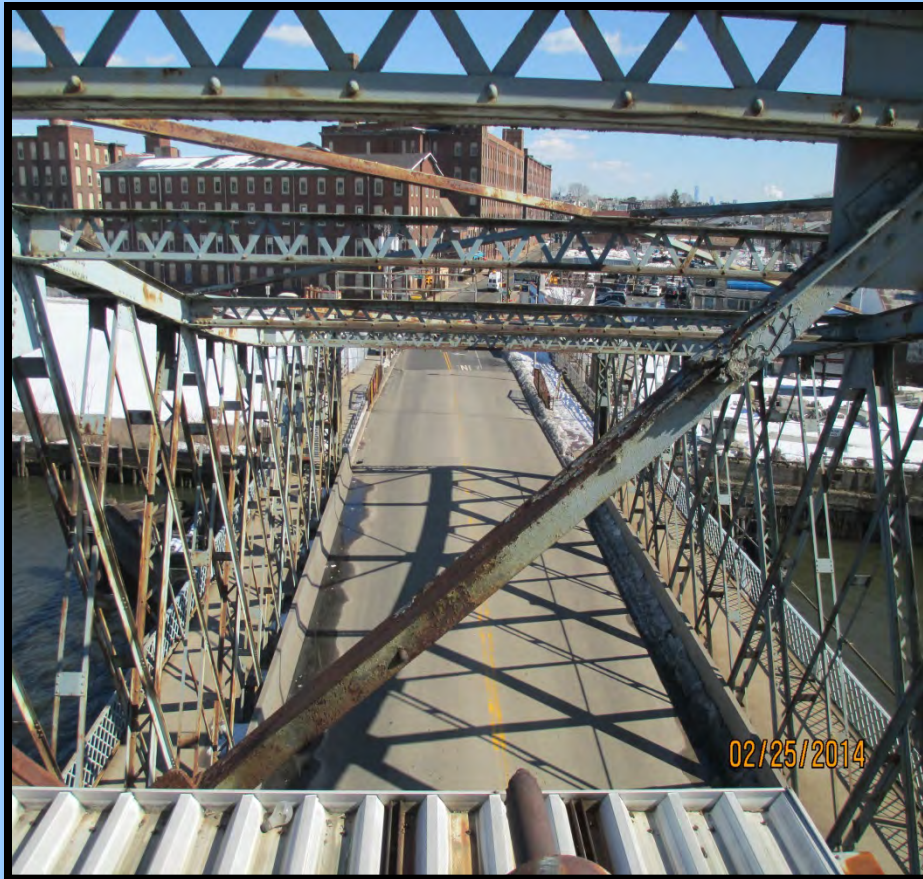
Photo 13: Localized rusting and material loss to top chords and diagonal truss members
