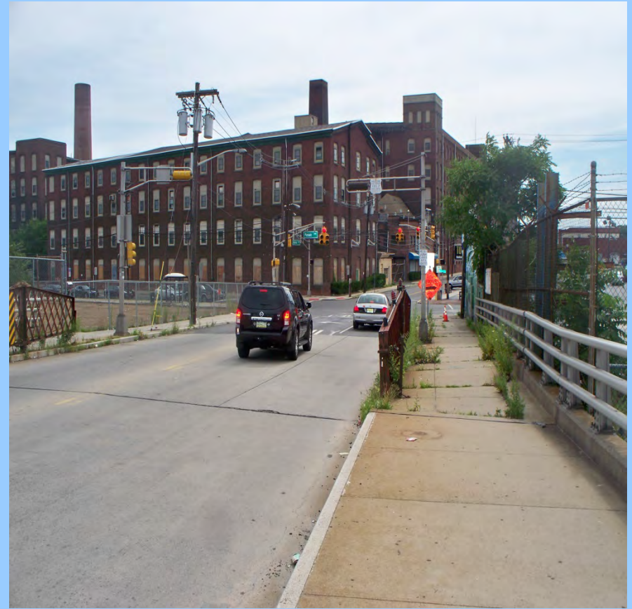
Photo 4: Looking east from bridge – substandard curb height on north side
