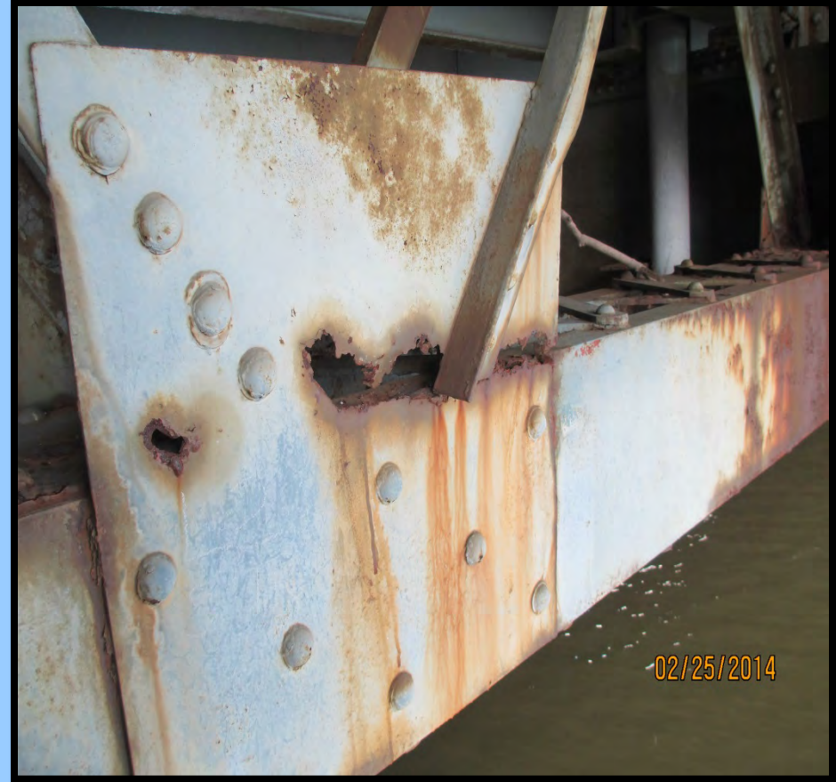
Photo 10: South truss gusset plate, severe rust with section loss
