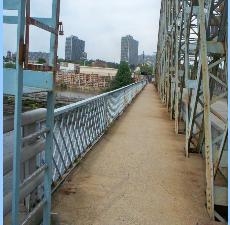
Photo 8: Substandard bridge railing
