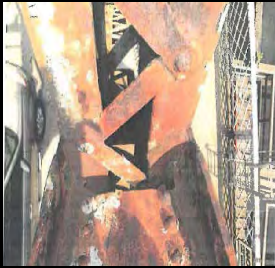
Photo 11: South truss connection, material loss to member angles connection plates, and lacing bars
