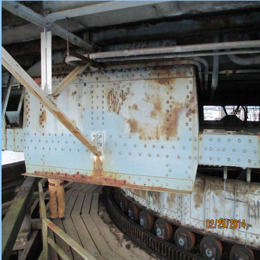
Photo 25: Rim bearing assembly of swing span – fair condition with corrosion build on exposed surfaces
