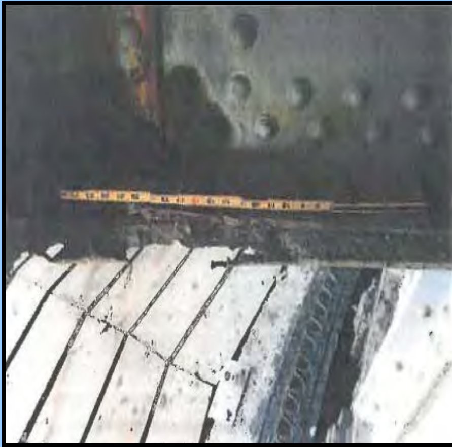
Photo 17: Section loss in bottom of support girder in swing span
