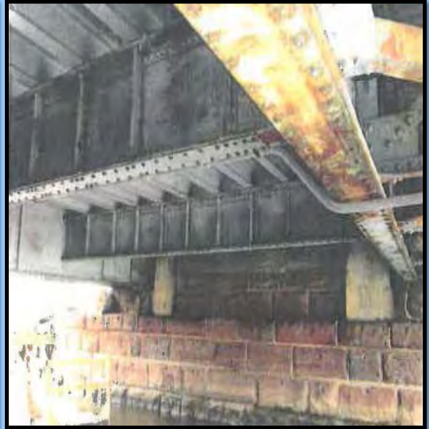
Photo 20: Rusting and localized section loss in girders and floor beams of west approach span
