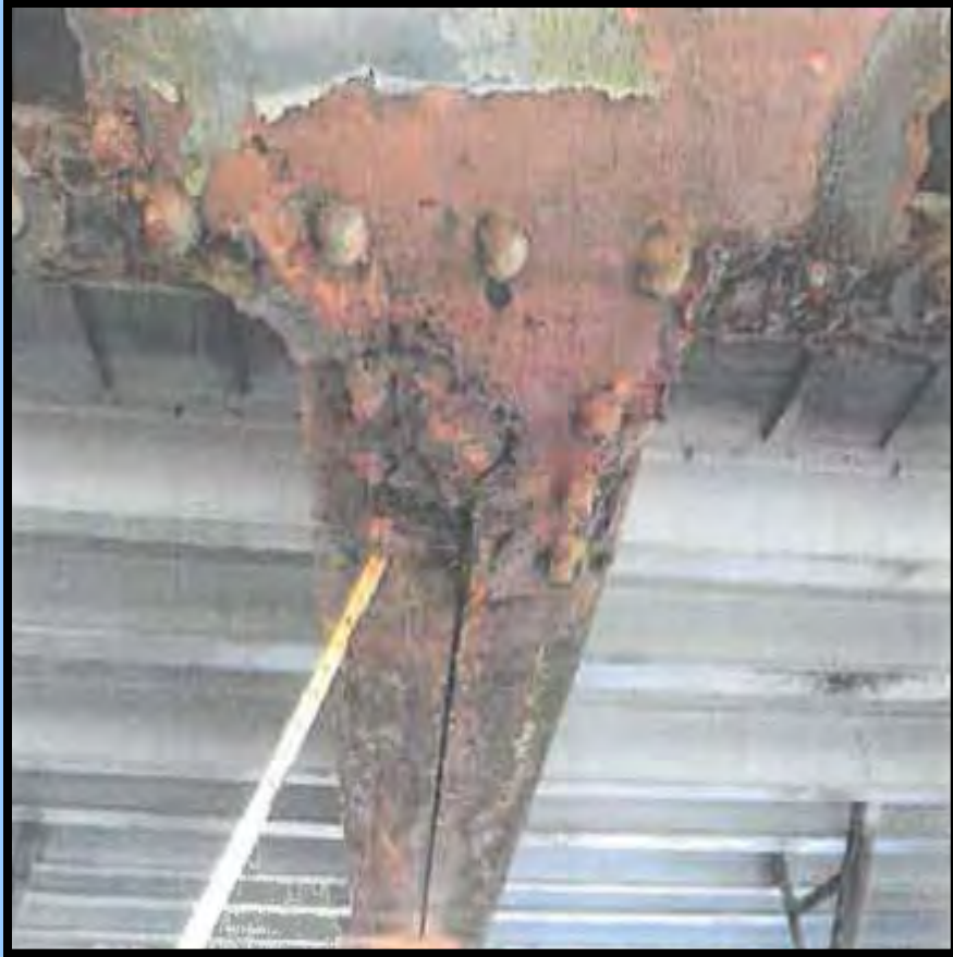
Photo 9: South truss bottom chord , severe deterioration to gusset plate, heavy rust throughout connection
