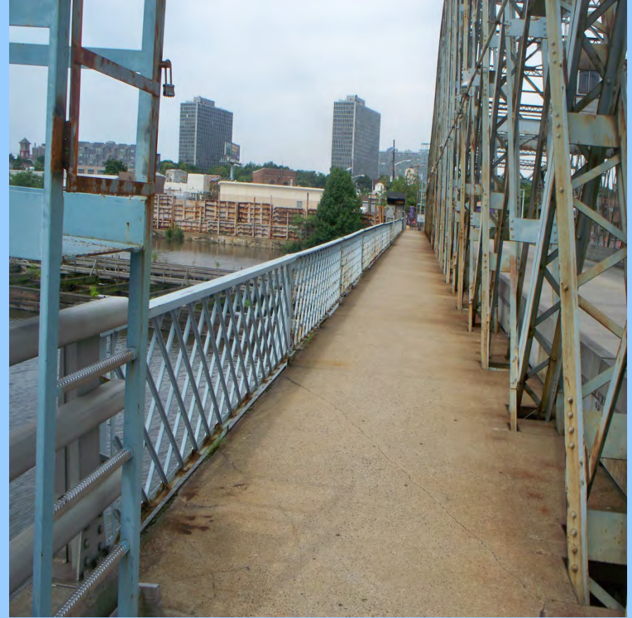
Photo 8: Substandard bridge railing
