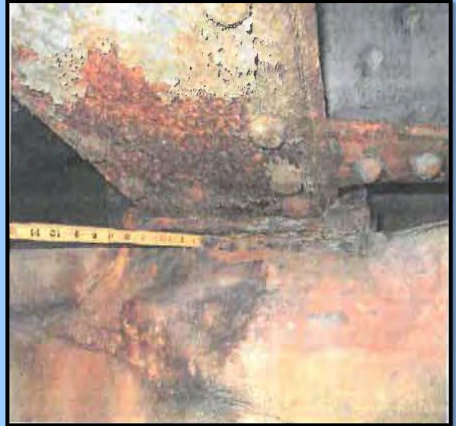
Photo 24: Undermining of south interior girder at west abutment
