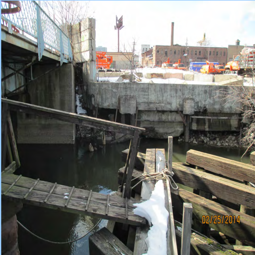
Photo 23: Northwest approach embankment undermining
